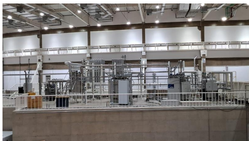
Figure 4: Cryogenic plant located above the accelerator tunnel near the RF cavities.
